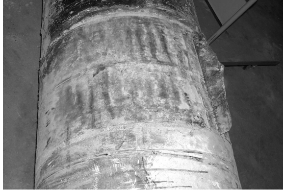
Figure 2. Wrinkles at the field applied coating
