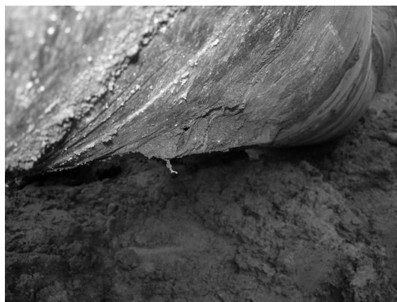
Figure 1. Coating failure at the field applied coating
